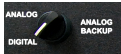
Figure 30: Analog Backup Switch
