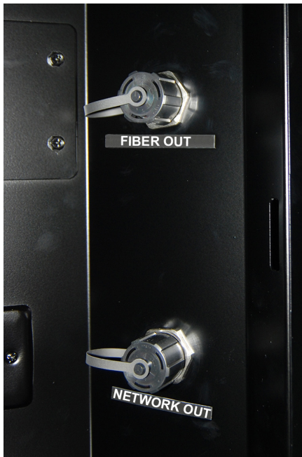
Figure 19: Left Connections (Rear View)
