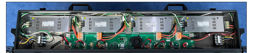
Figure 40: Power Supplies in Power Box
